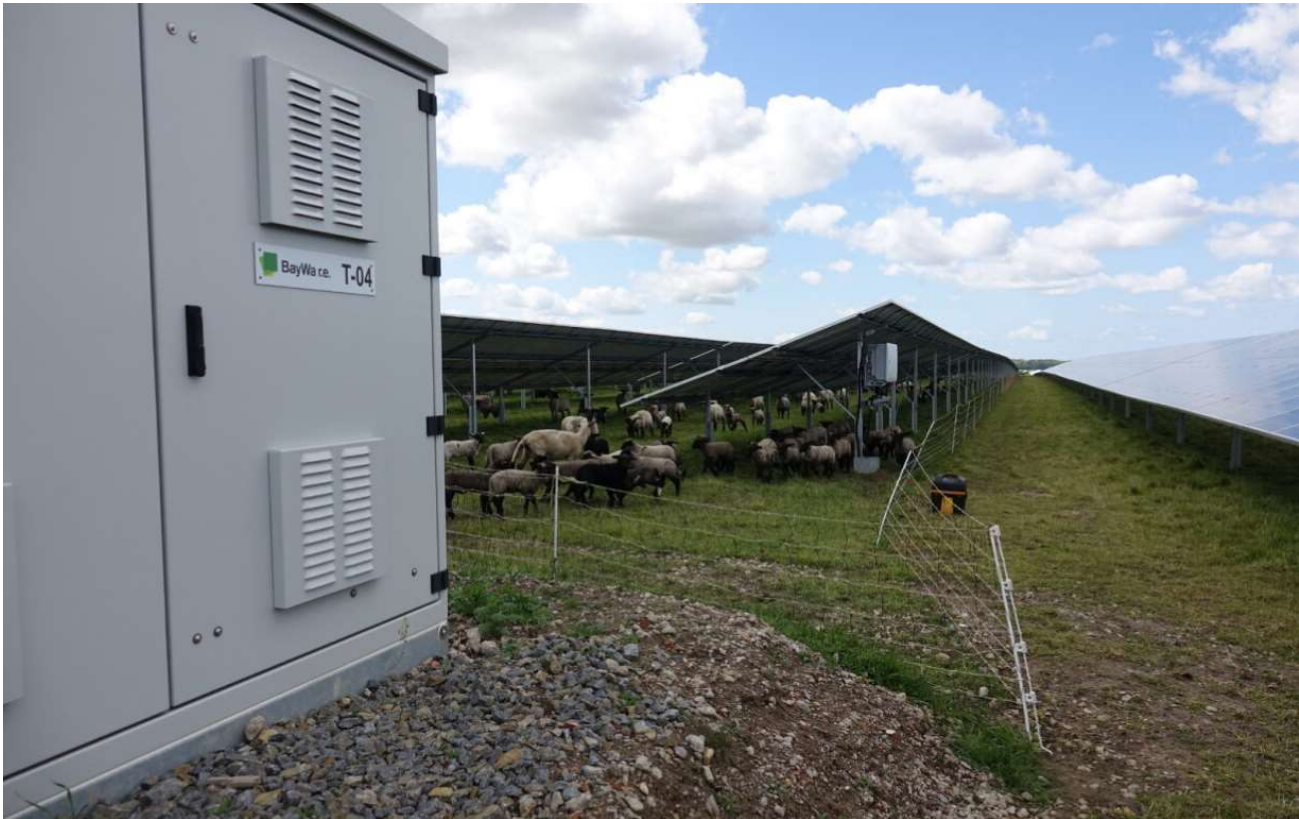
Plate 3: Typical transformer on a solar farm site
